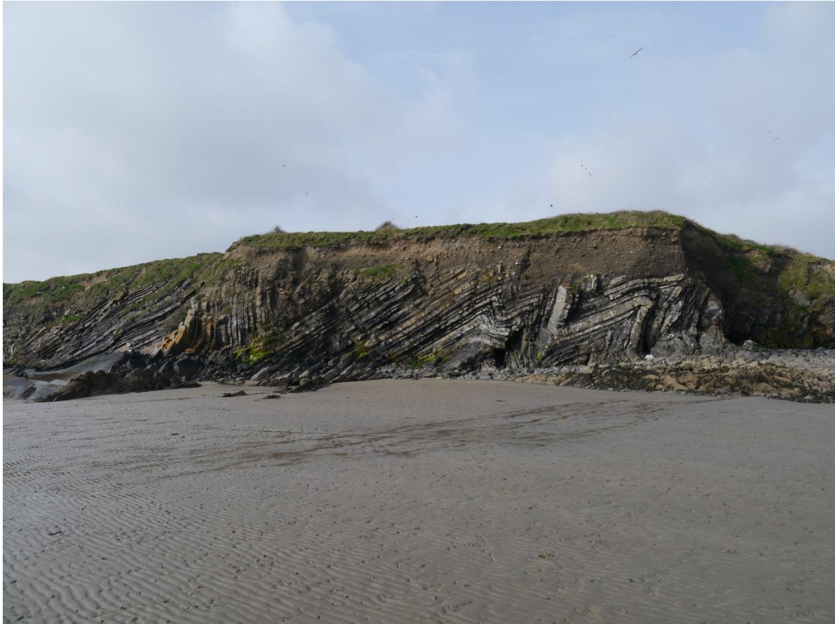
Fig. 7 Coastal section at Loughshinny, Co. Dublin showing chevron folds of Brigantian age (photo by David Chew)
